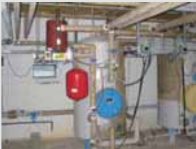
Hot water storage for the solar heating system at Aabenraa Hospital (Denmark)
