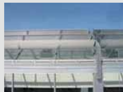
Solar shading of glazed courtyard at Aabenraa Hospital
