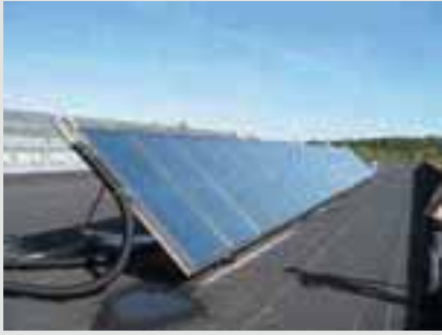
Solar heating system on the roof at Aabenraa Hospital (Denmark)
