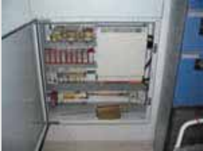
BEMS unit at Aabenraa Hospital (Denmark)
