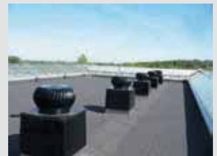
Roof integrated wind cowls at Aabenraa Hospital
